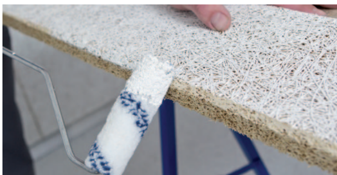
Painting the bevel - Use a brush or a thin paint roller to apply the paint.
